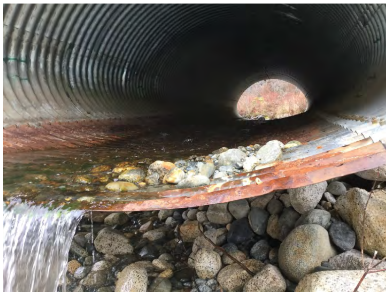
Culvert is sagging where unsupported at outlet
