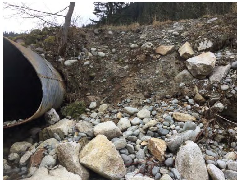
Downstream left fillslope eroding
