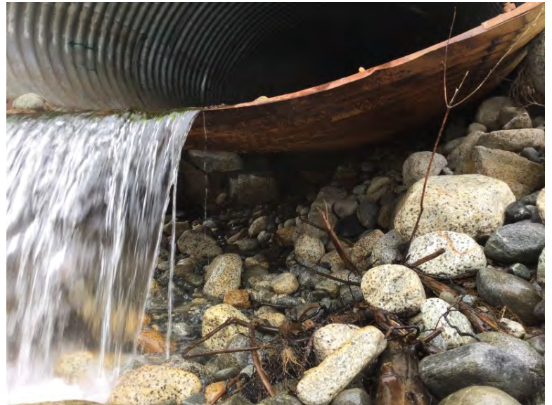
6m of outlet culvert unsupported
