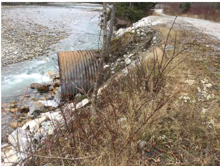
Downstream left fillslope eroding and over steepened at 1.25:1
