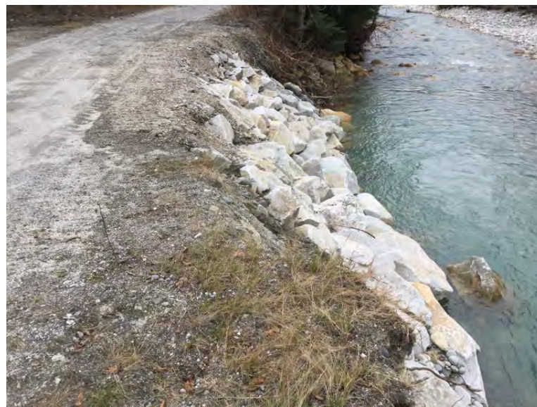
Fillslope repair 30m from culvert
